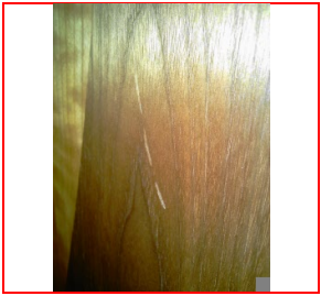
Door Finish - scratched
