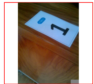
Cabinet - chipped (to front face)
